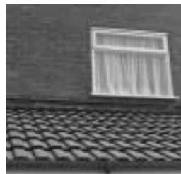
Type E cavitrays used with a lead flashing, where a new roof abuts an existing wall.
